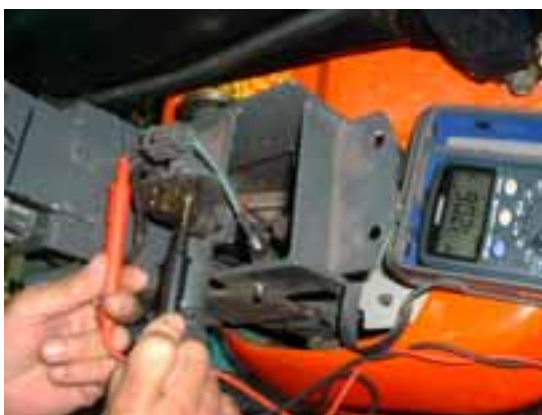
(Battery 12V test : Key switch is on)
